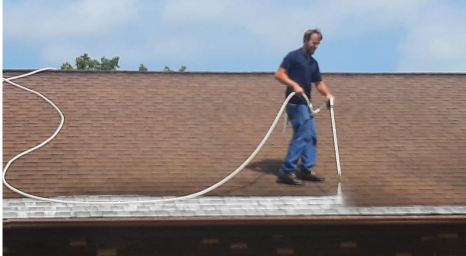
Luke Meyer of Biobased Spray Systems, LLC, Applying RoofRestor Photo Credit: Harold Stanislawski, AURI
