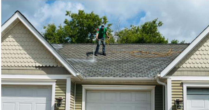
Roof Maxx Soy Roof Rejuvenate Demonstration, Thief River Falls, MN Photo Credit: Jaime Schad, Shingle Revival by Roof Max
