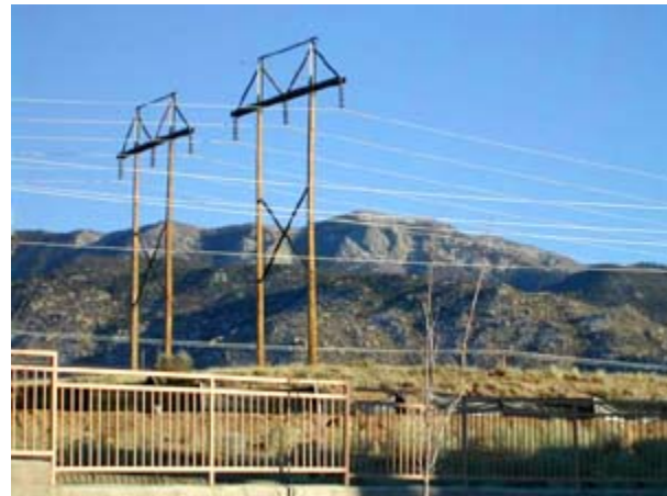
230 kV transmission line. Notice the three wires or conductors hanging from each tower. Three or four wires generally will signify a three phase transmission line. Picture source: U.S. Department of Labor: Occupational Safety and Health Administration
