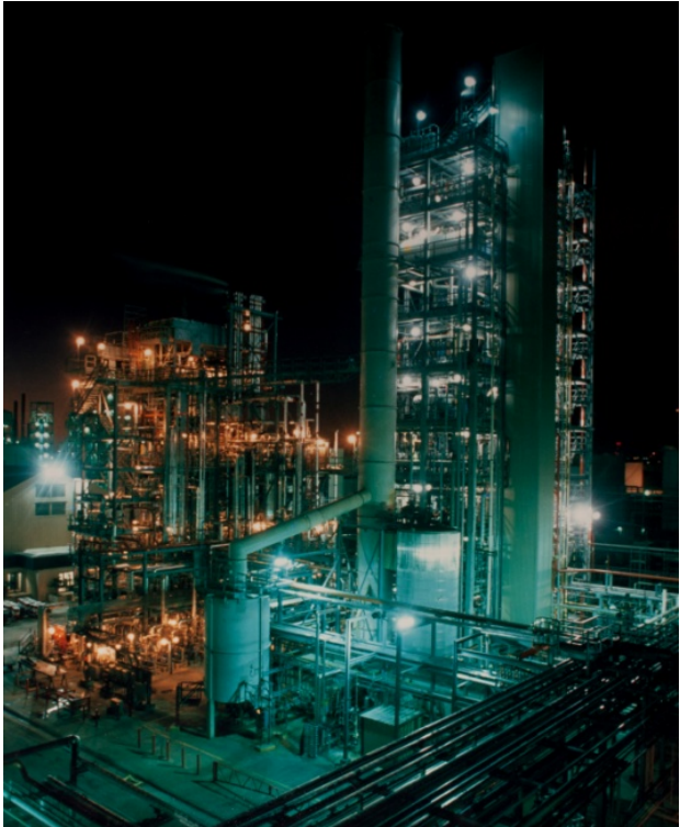
200 BBL/Day Gasifier Island & FT Diesel PDU at Exxon Baton Rouge Refinery
